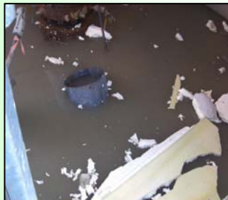
SSV housing (at rest) along with insulation
