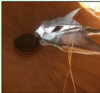
Impact at well house ceiling
